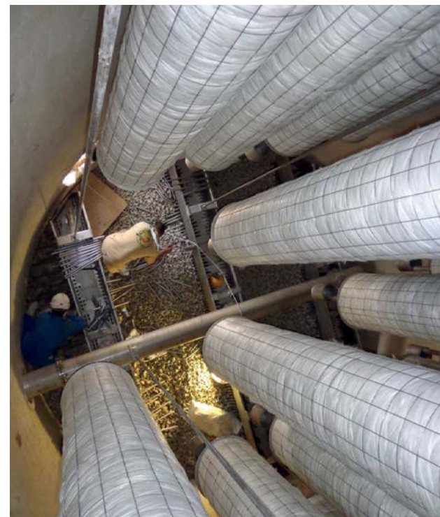
A view of the MECS® Brink® mist eliminators in the new acid tower.
