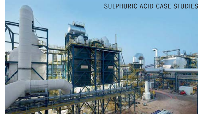
Mazidagi's gas cleaning plant section.
