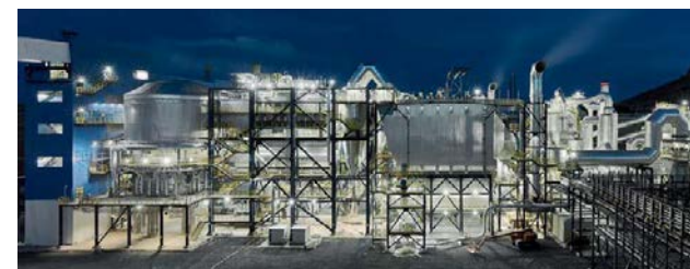
Mazidagi's roasting-gas cleaning-acid plant sections.
