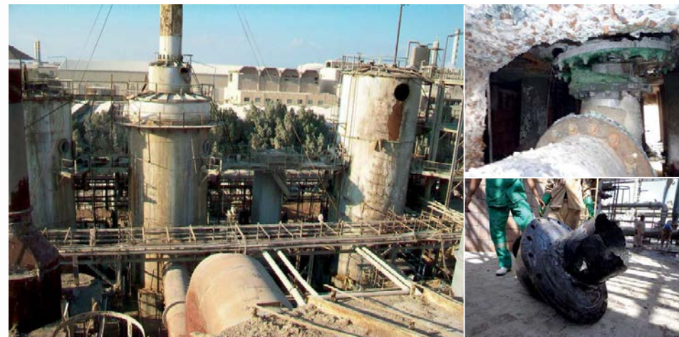
Above left: AZFC's Unit 6 before the revamp – the drying and absorption towers were in very bad shape. Above right (top and bottom): Acid was leaking from the bottom of the acid tower, causing corrosion issues.
