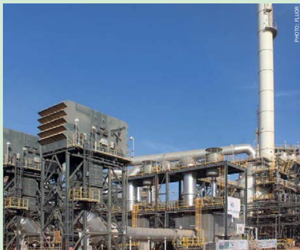
MWSPC sulphuric acid plant.
