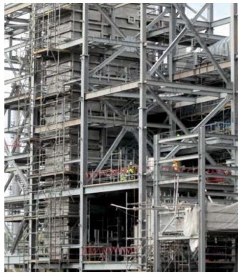
Fig. 7: Construction phase of a rectangular modularized MMV scrubber installation for a 1,000 t/d urea granulator.
