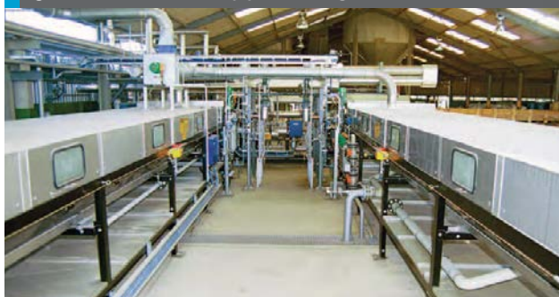
Fig 6: Rotoform skid-mounted equipment showing hood
