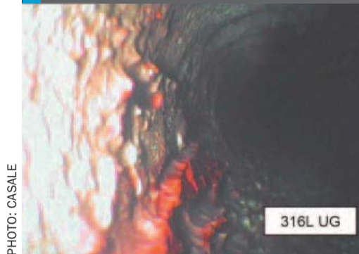
Fig 1: Active corrosion on stainless steel
