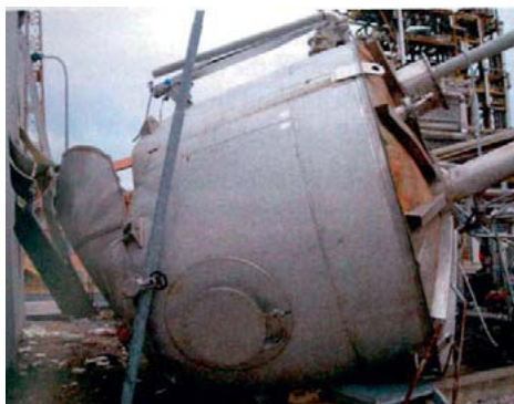
Fig. 10: Ruptured aqueous ammonia storage tank, Europe, 2009.
