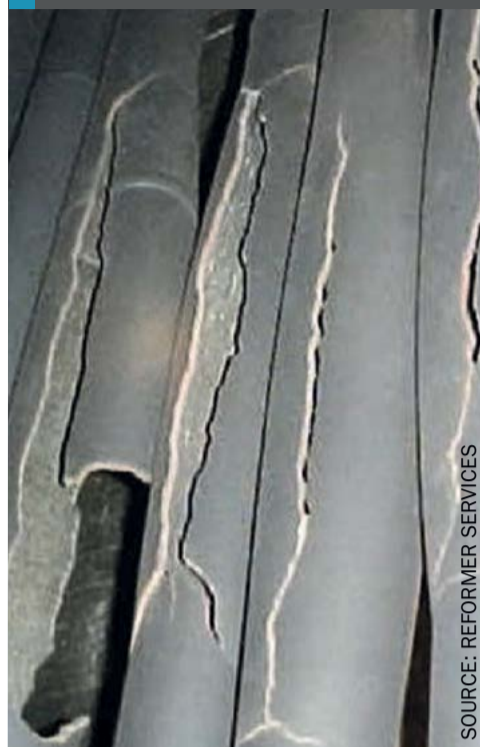
Fig. 18: Crack in reformer tube
