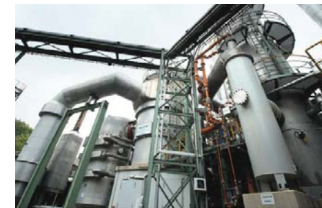
Fig. 4: CORE™ add-on system in operation.
