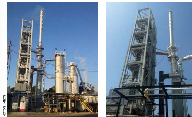
Fig. 10: Southern States commercial SolvR® plant.
