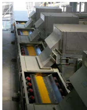
Discharge of sulphur pastilles from steel belt cooler.
