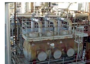
Fig. 1: Electric reheaters (upper part visible above platform) installed in revamped SRU.
