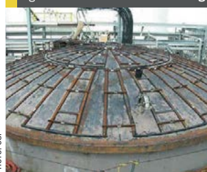
Fig. 4: ControTrace tank roof heating
