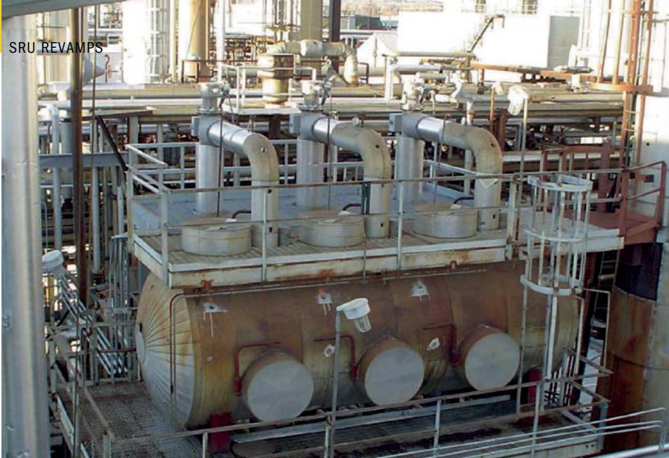
Electric reheaters installed in a revamped SRU to replace an underperforming hot gas bypass system (upper part of reheaters visible above platform). PHOTO: WOOD
