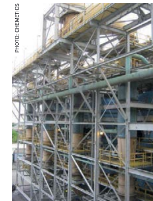
Fig. 3: Chemetics wet gas condenser.
