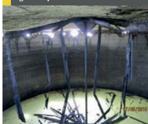
Fig. 3: Sulphur tank structure corrosion
