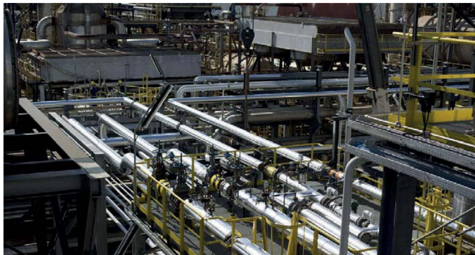
Sulphur recovery unit in Turkey.
